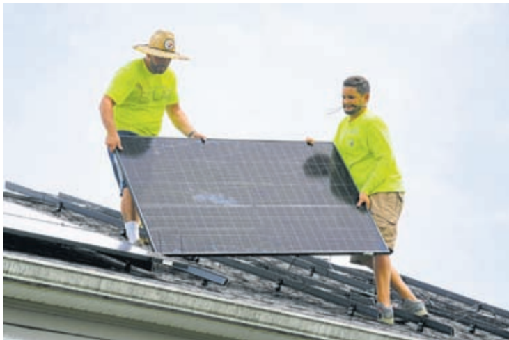
Even Berrios, left, and Nicholas Hartnett, owner of Pure Power Solar, install a solar panel on the roof of a home in Frankfort, Ky., July 17, 2023.
